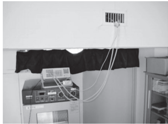
d) Heating duct in the lab. in the college
