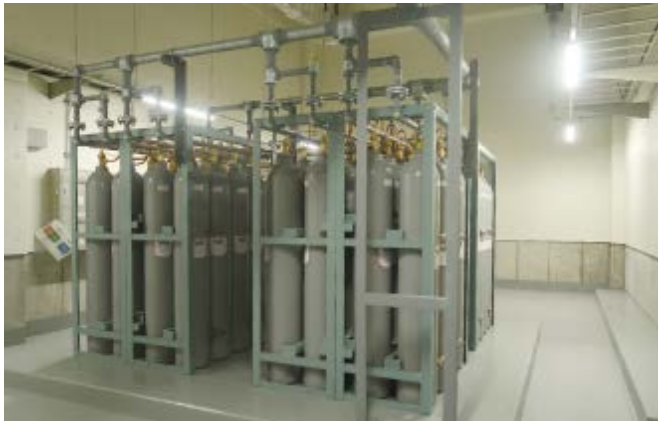
Fire extinguishing equipment using nitrogen gas
