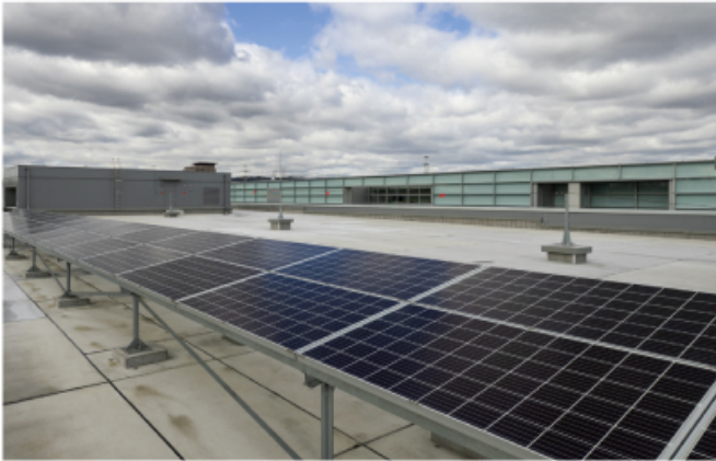
Solar power generators on the roof top
