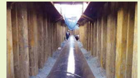
Japan Water Agency / Toyogawa Canal Second Stage Project / Eastern Main Canal Parallel Channel / Tahara City, Aichi Prefecture
