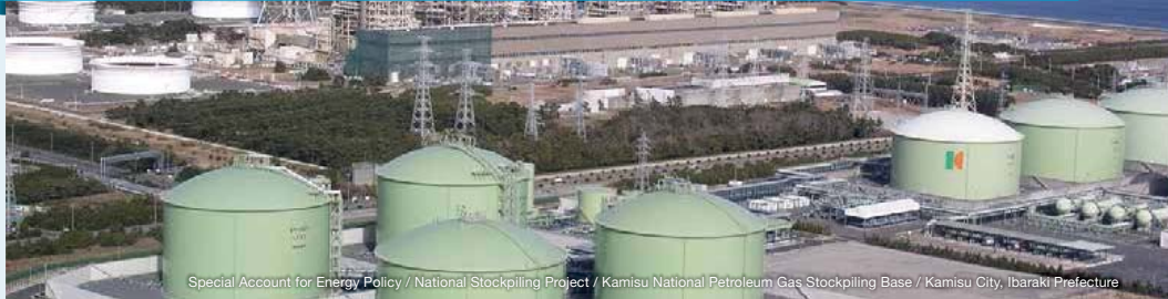
Special Account for Energy Policy / National Stockpiling Project / Kamisu National Petroleum Gas Stockpiling Base / Kamisu City, Ibaraki Prefecture
