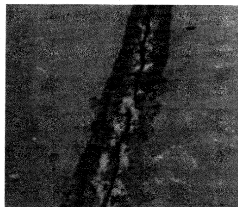
Photo 1 Thermal Crack of Asphalt Layer
