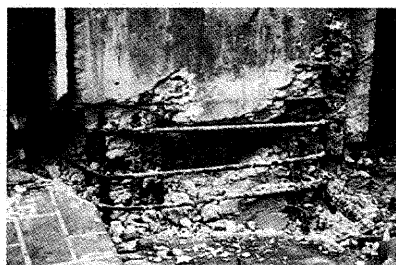
Photo 1 被害状況 (Damage of SRC Column Bases)
