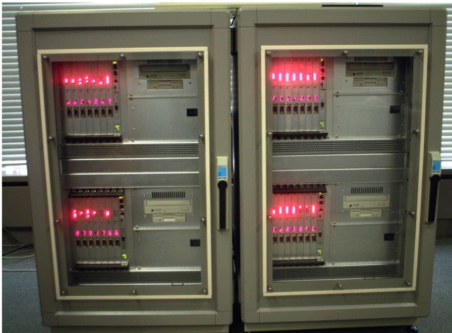
Figure 3. Front view of the four EHPC units system.
