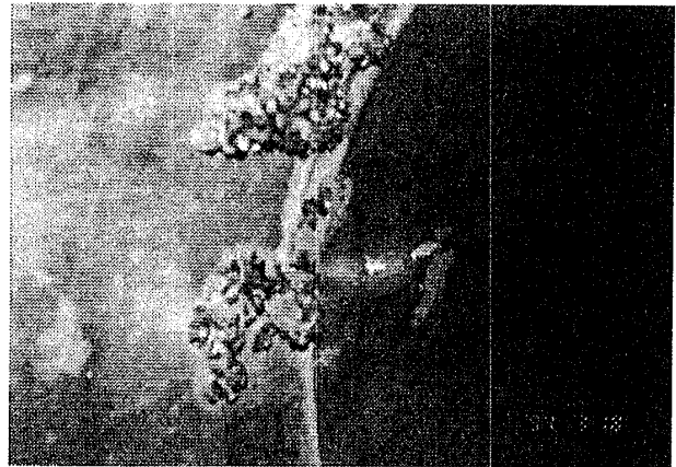
Fig. 11 The antifouling state by the antifouling system undertaken for the steel sea water pipe in Y power plant (B part) (H6.3.18)
