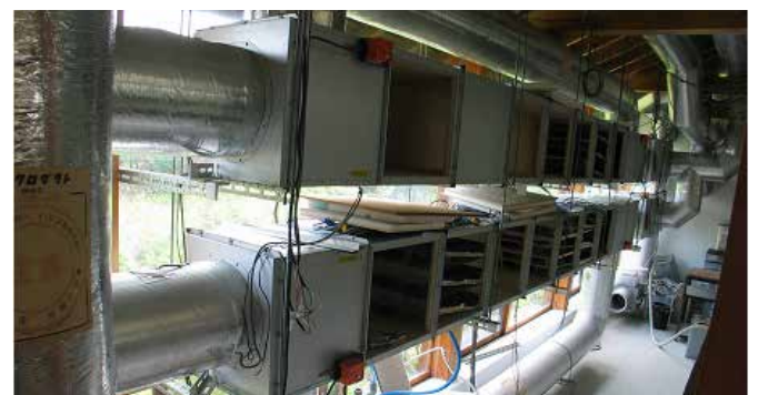
Upper: Heat collection testing facility measuring and comparing energy conservation under changing building and equipment conditions.
