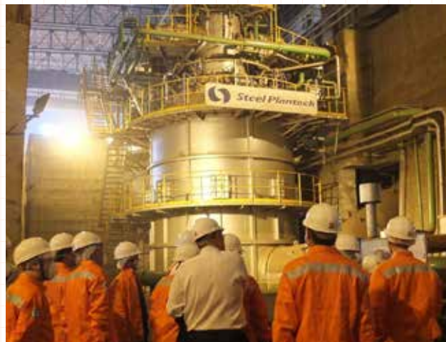
Completed test facility for the "Environmentally Conscious High-Efficiency Arc Furnace Demonstration Project" in Thailand (combustion tower inside the exhaust gas treatment facility)
