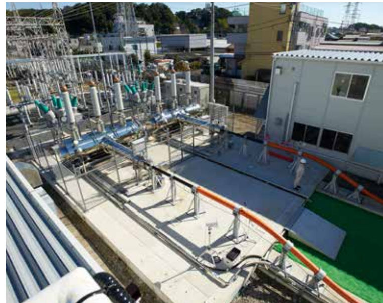
Demonstration test of a superconducting cable at Tokyo Electric Power Company, Incorporated's Asahi substation.
