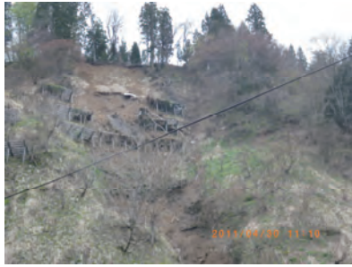
図14 地震によって崩壊した雪崩予防柵(新潟県十日町市) Fig.14 Collapse of avalanche supporting structures due to the earthquake.
